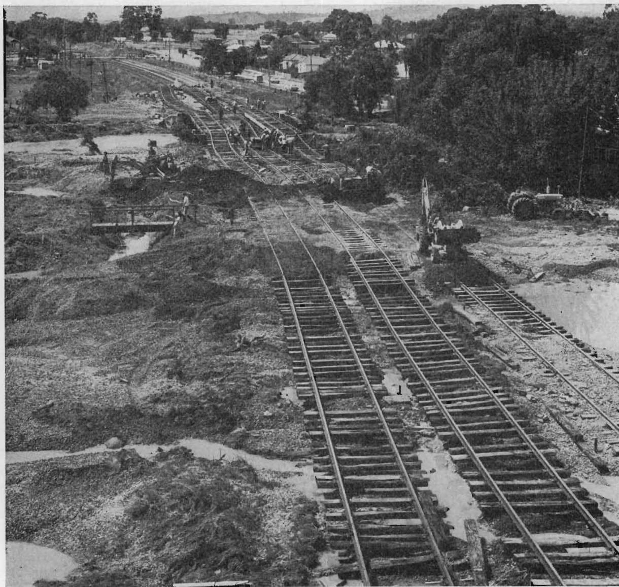
Flooding at Seymour in February caused severe damage to the main Melbourne to Sydney rail tracks. The standard gauge track is on the right.
